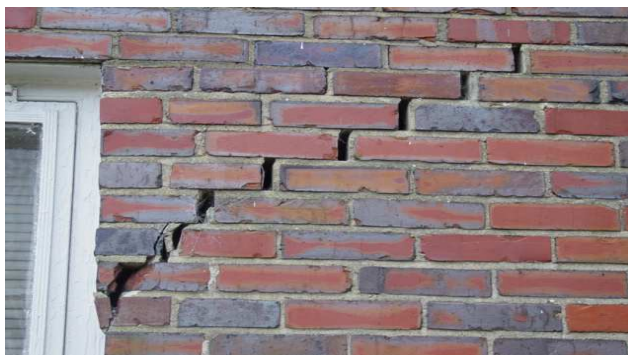
A view of diagonal cracks in the exterior brick wall.
