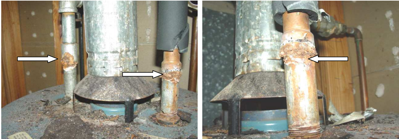
A wide angle view and a close up view of the corroded water supply pipes.
