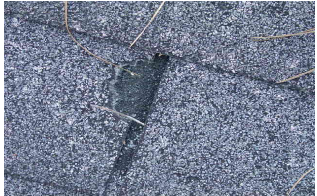
A view of hail damage.
