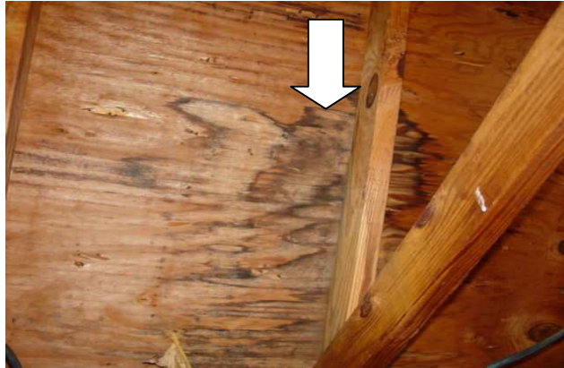
A view of moisture stains on the roof decking.
