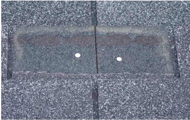
A view of a torn shingle tab.
