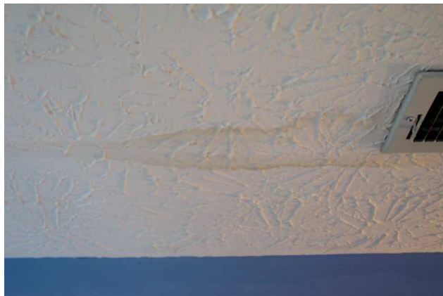
A view of a ceiling stain in the upstairs bathroom.
