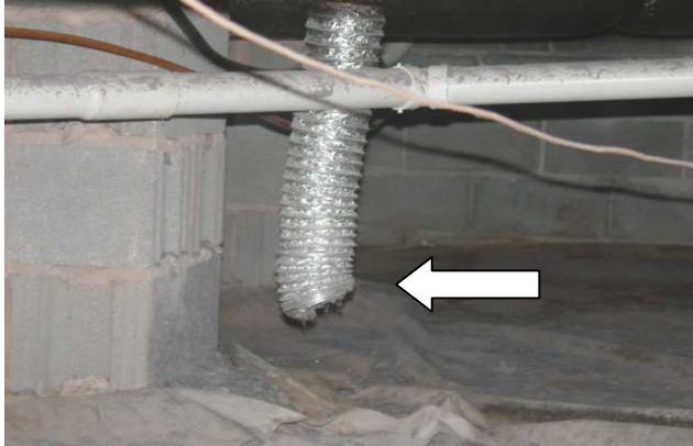
A view of a dryer vent terminated inside the crawl space.
