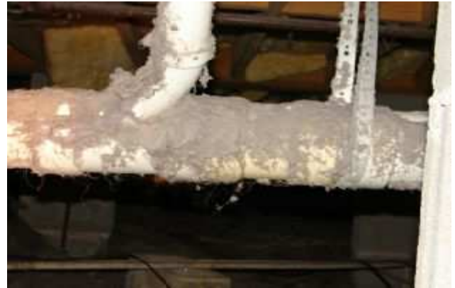
A view of lint build-up inside the crawl space.
