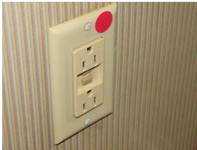
A sample view of a faulty GFCI.
