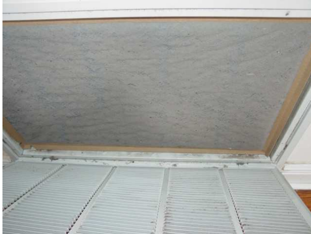
A view of one of the clogged filters.
