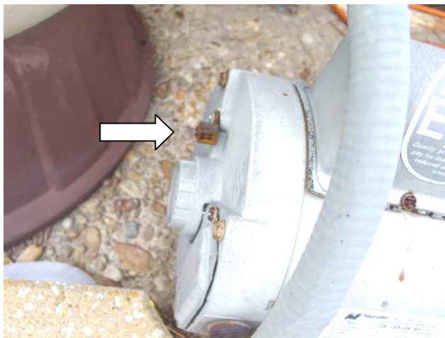
A view of the missing bond wire from the bond clamp.
